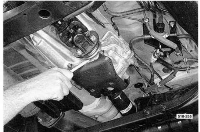
Check the transfer case output shaft seals for leakage.
