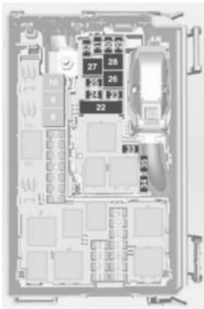
Vauxhall Meriva B – fuse box – engine compartment
