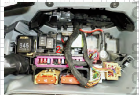
Relay and fuse carrier in E-box
