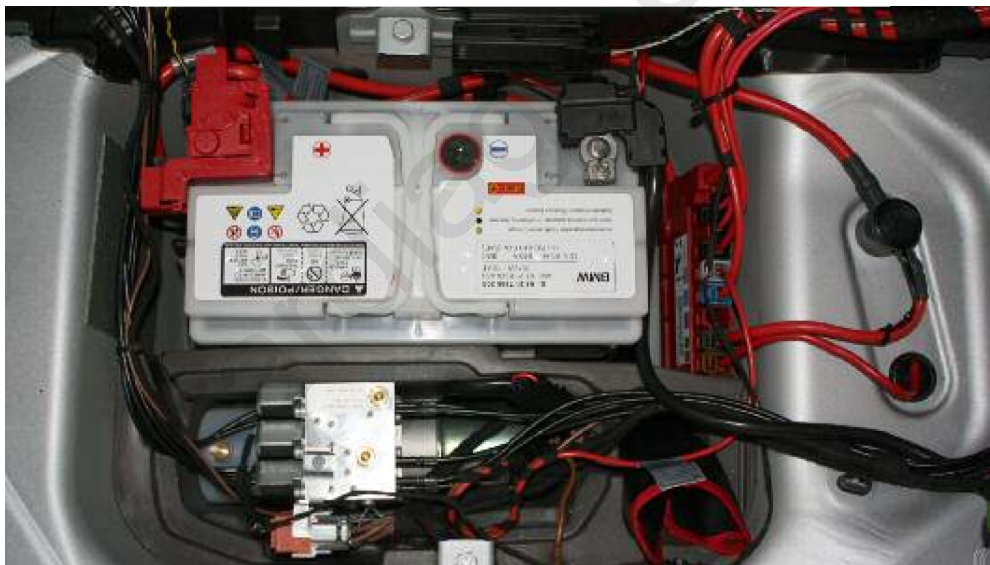
Hydraulic Unit Location
